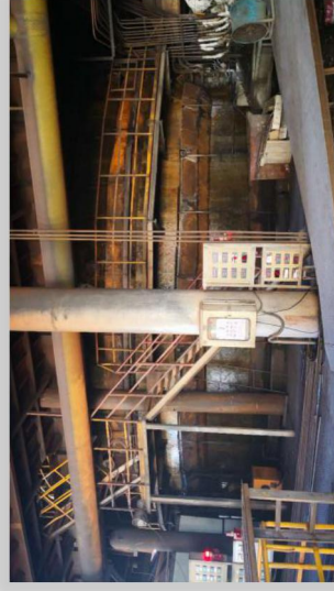
矿热炉 Ore Furnace
